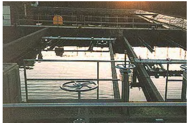
Primary Clarifier/Settling Tank
