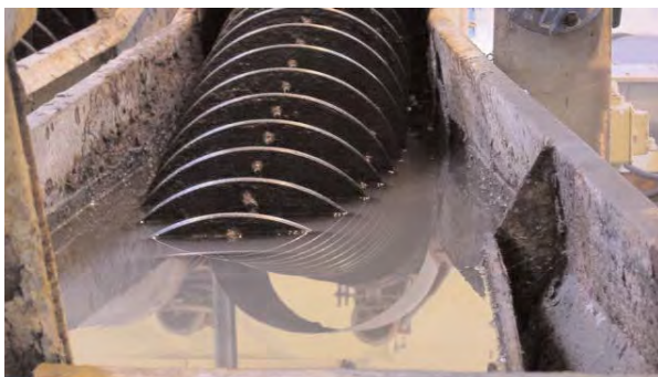
Screw Conveyors used for Grit Removal
