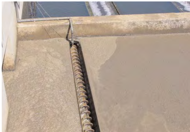
Scum Collector with travelling conveyor
