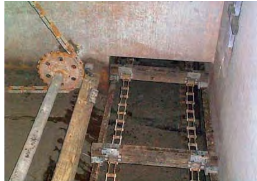
2 systems of grit chamber scraper apparatus applications
