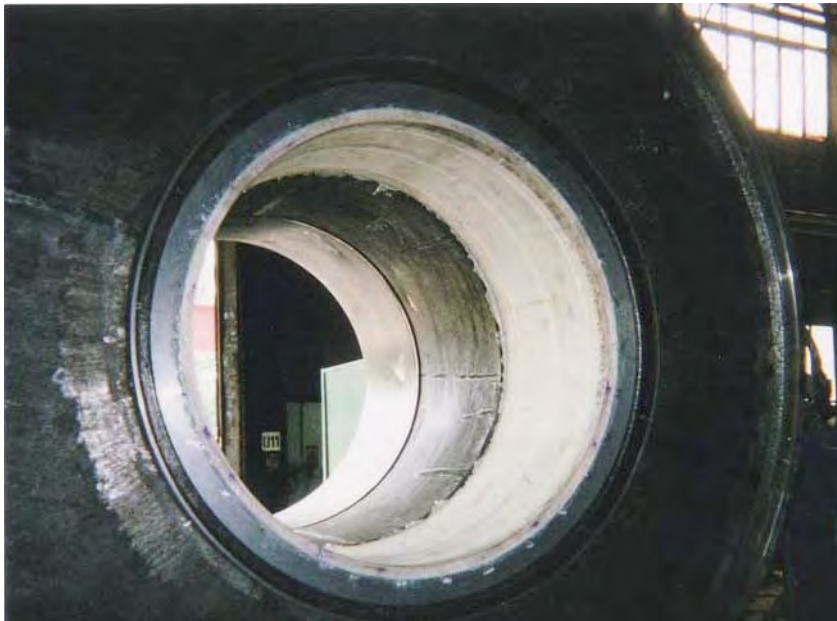
Thordon SXL bearing installed
